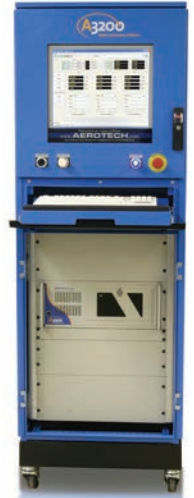
Advanced Control Systems
